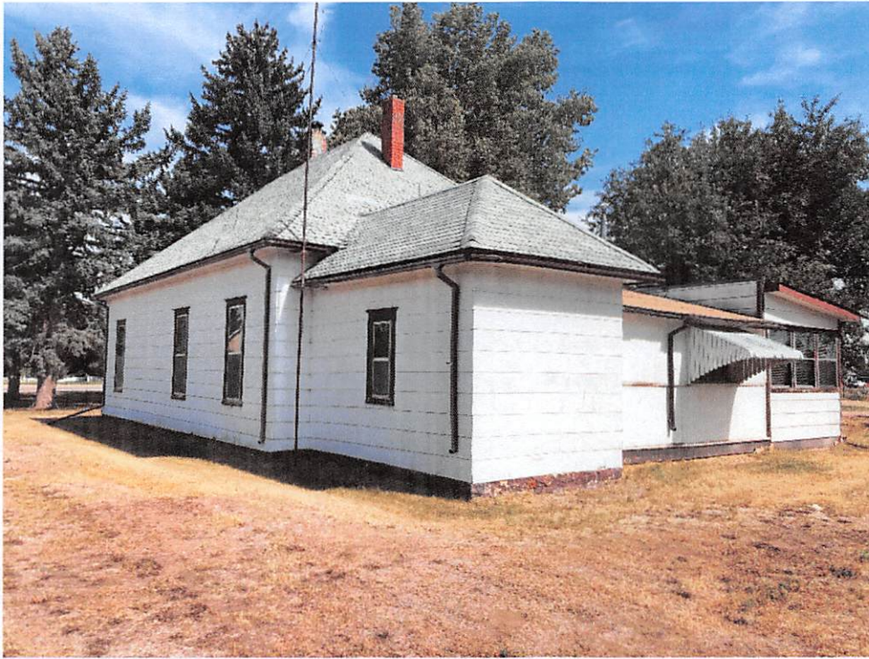
West side of the house showing first addition along with subsequent later additions. These were done with lower quality materials and are not as structurally sound.
