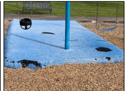
Surfacing repair needs
