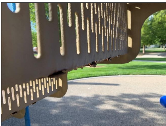
Playground stair joint
