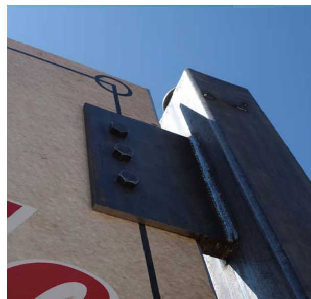
WEATHERED STEEL POST, BRACKET AND FASTENERS
