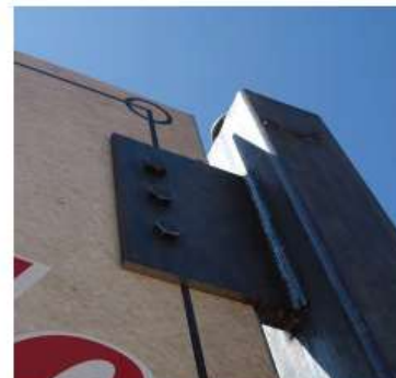
WEATHERED STEEL POST, BRACKET AND FASTENERS
