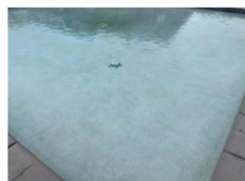
Figure 26 Surface staining and discoloration
