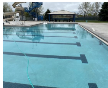
Figure 5 Pool surface staining, etching
