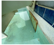
Figure 14 Corrosion on supply grate
