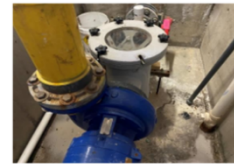
Figure 21 Pool pump and strainer
