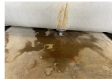
Figure 23 Leaking pool filtration
