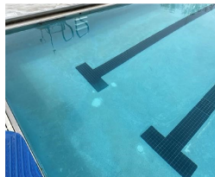
Figure 2 Plaster patches on pool surface
