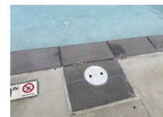
Figure 27 Cracking through skimmer basket
