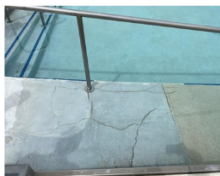
Figure 4 Surface cracking on entry ramp
