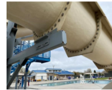
Figure 18 Waterslide support beam corrosion
