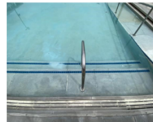
Figure 3 Delamination and cracking on pool entry stairs
