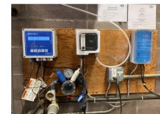
Figure 30 Children's pool chemical automation
