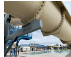
Figure 18 Waterslide support beam corrosion
