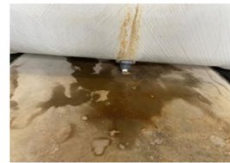
Figure 23 Leaking pool filtration
