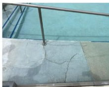
Figure 4 Surface cracking on entry ramp
