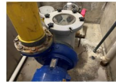
Figure 21 Pool pump and strainer
