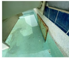
Figure 14 Corrosion on supply grate
