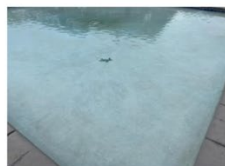
Figure 26 Surface staining and discoloration
