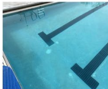
Figure 2 Plaster patches on pool surface
